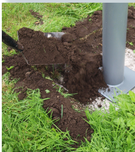
Make sure the fitness station is stabil and properly fastened before filling with dirt to the ground line.
